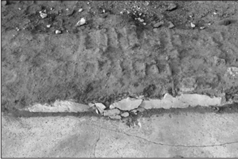
Fig. 5. Plaster on the southern face of the north wall of unit B.22 (Photo W. Godlewski)
