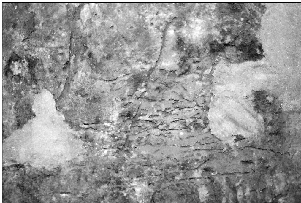
Fig. 4. Face of mural from the Lower Church (after application of putties and preliminary reinforcing of the plaster structure), demonstrating a full gamut of damages: termite tunnels, white spots of salt crystallization – chiefly gypsum, black fungi (?) colonies (Photo D. Moryto-Naumiuk)
