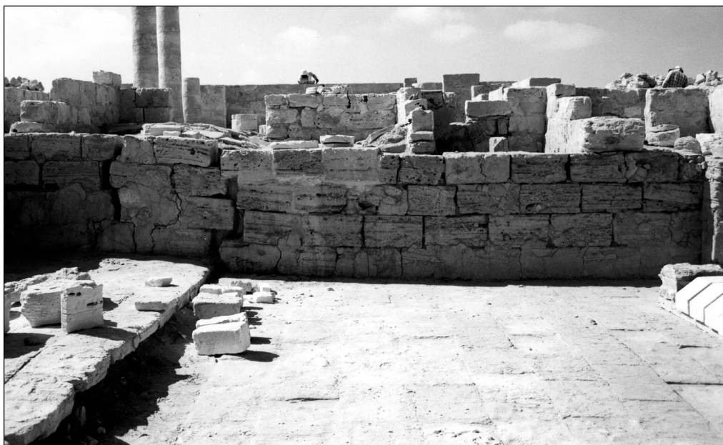
Fig. 5a. Hall H 21 "N". Before conservation. Close-up view from the north of the cracked south wall and displaced pavement (Photo S. Medeksza)
