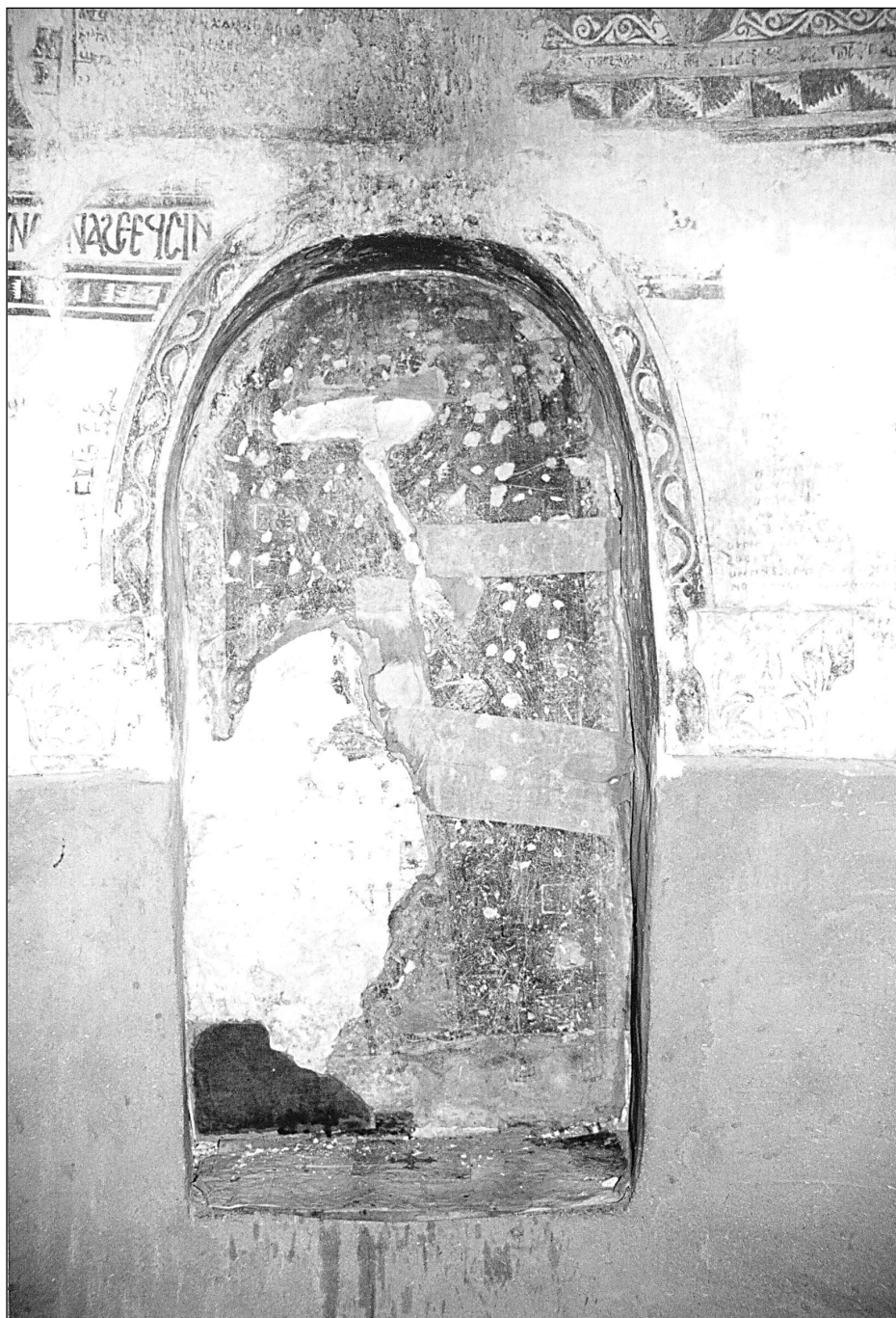
Fig. 1. Wall-paintings in the central niche of the church apse, before conservation (Photo C. Calaforra-Rzepka)
